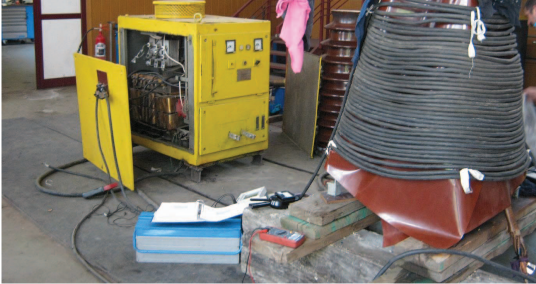
Fig. 1. Detail about the drying of current transformers in actual technology.
