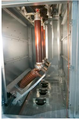
Fig. 12. Assembly of HBC fuses and in the upper part LBS
