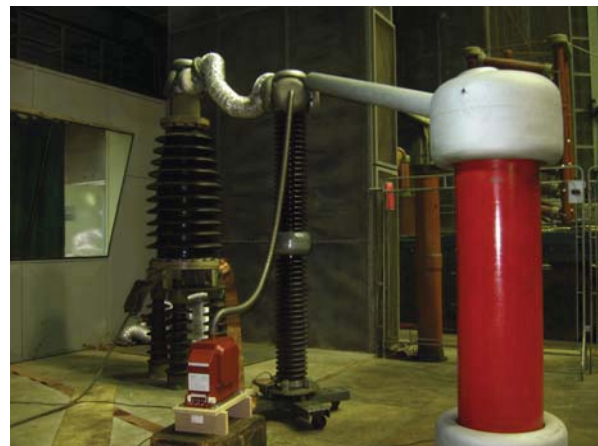
Figure 9: PD measuring circuit at a 20\sqrt{3}/0.1/\sqrt{3}/0.1/3V voltage transformer
