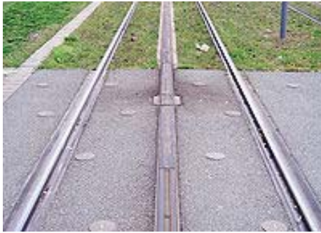
Figure 1. Rail with APS system
