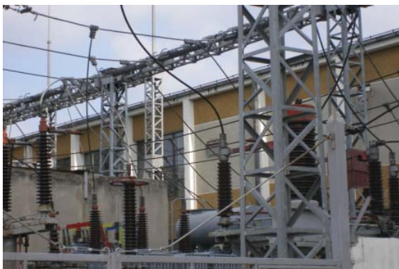
Fig. 1. Power distribution facility
