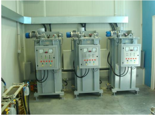
Fig. 5. Voltage regulating autotransformer group - three single-phase units.
