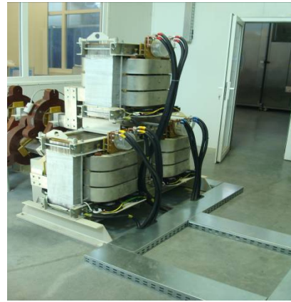
Fig. 7. Final power transformer group - three single-phase units
