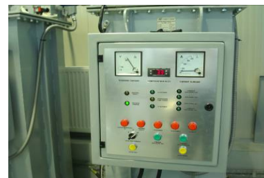
Fig. 4. Local autotransformer control and protection box.
