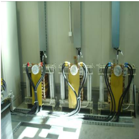
Fig. 6. Intermediate power transformer group - three single-phase units.
