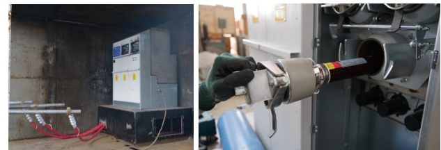
Fig. 12. Distribution switchgear in experimental circuit for pressure testing. Fuse placement on a side phase.
