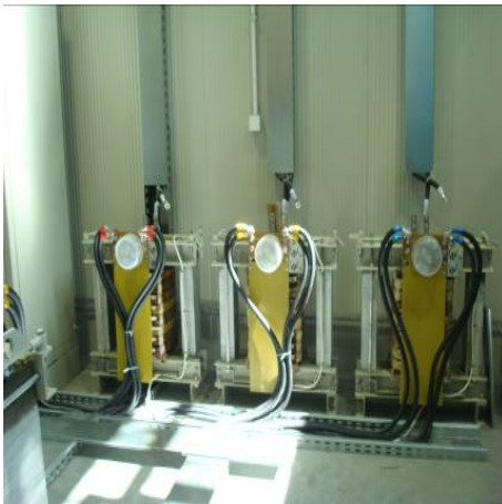
Fig. 6. Intermediate power transformer group - three single-phase units.
