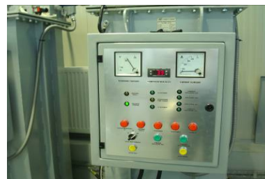
Fig. 4. Local autotransformer control and protection box.
