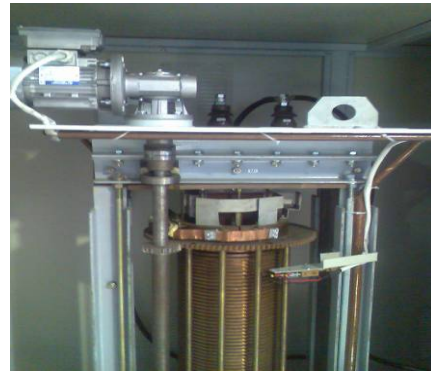
Fig. 3. Internal structure of the autotransformer showing the flux divider and slip ring collector.
