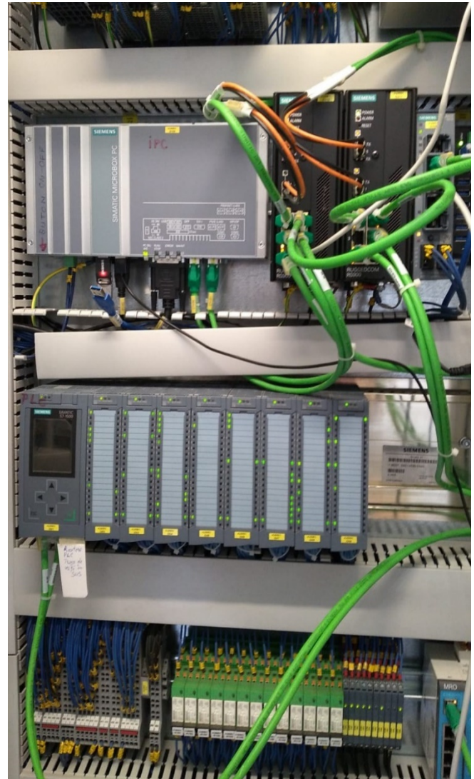
Fig. 3. PLC in the SCADA panel.
