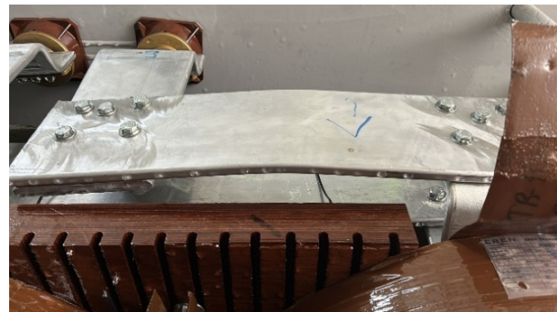
Fig. 20. Photo of the transformer after removal from the tank.
