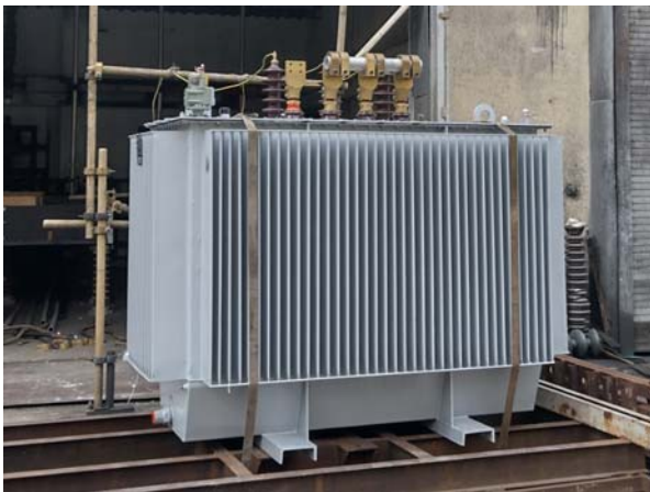
Fig. 18. Photo of the transformer used for experiments with short-circuited terminals.
