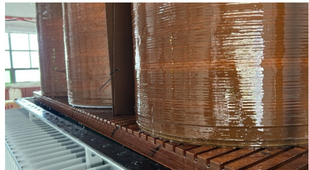
Fig. 21. Photo of the transformer after removal from the tank.
