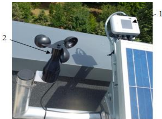
Fig. 4. Equipment for measuring weather parameters: 1- pyranometer; 2- anemometer.
