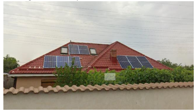
Fig. 12. Image of the PV panels mounted on the West facade of the roof (PV2 string)
